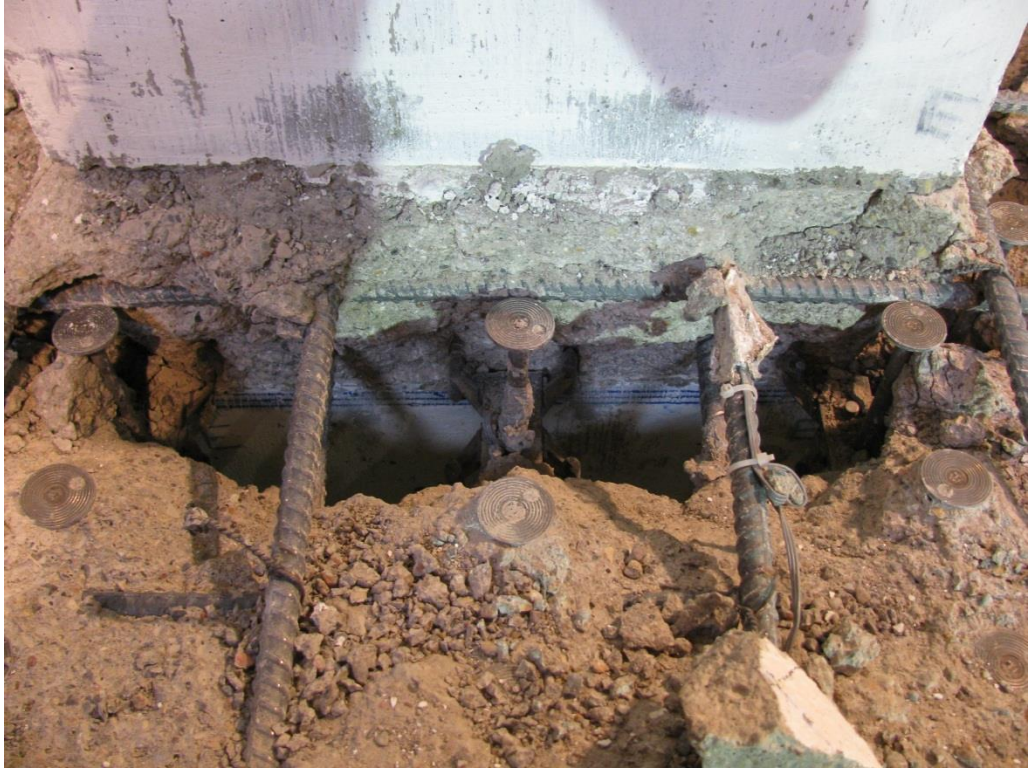
Figure 3-16: Specimen B2 – Connection Region where Severely Degraded Concrete was Removed by Hand After Test
