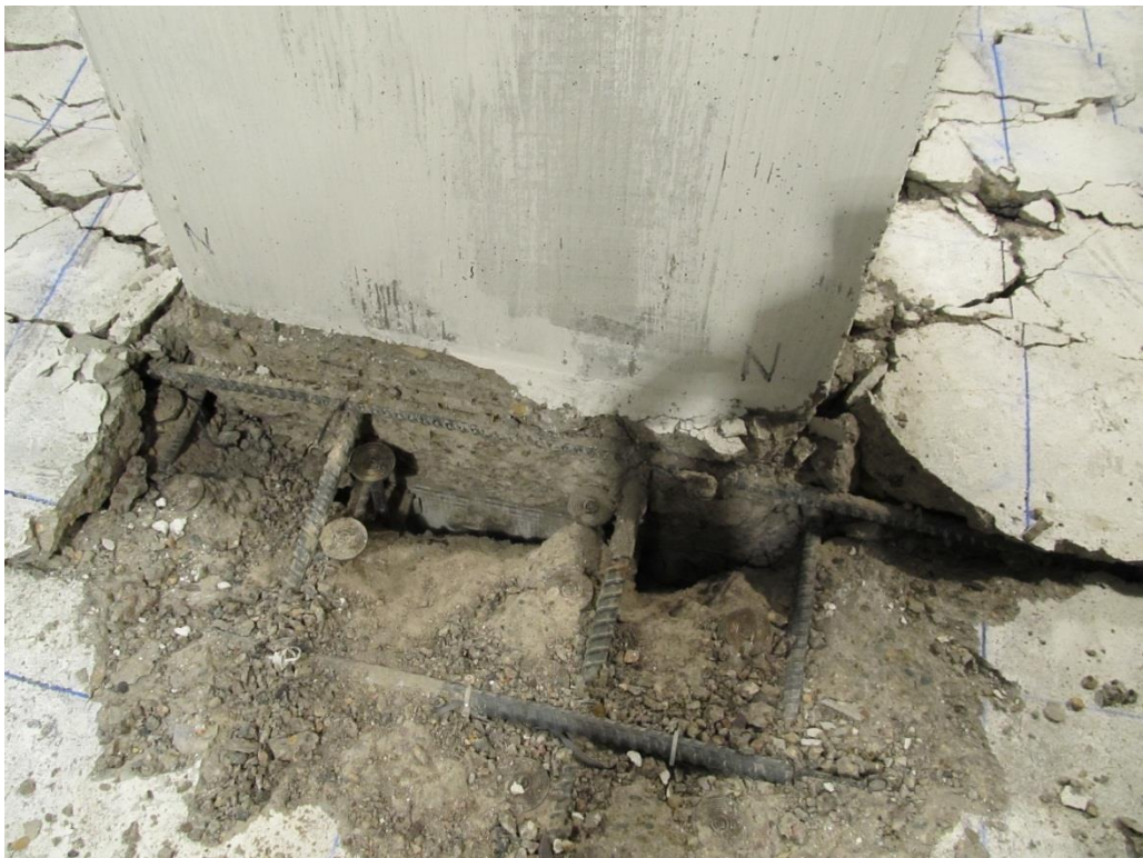
Figure 3-21: Specimen B4 – Void in Connection Region after Loose Concrete was Removed After Test
