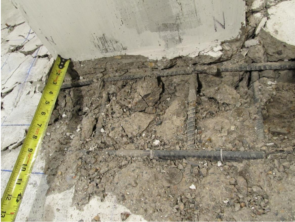
Figure 4-25: Specimen B4 – Gravel-Like Concrete within Connection Region
