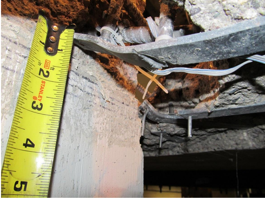
Figure 3-22: Specimen B4 – Bending of Base Rail on South-East Face of Column After Test
