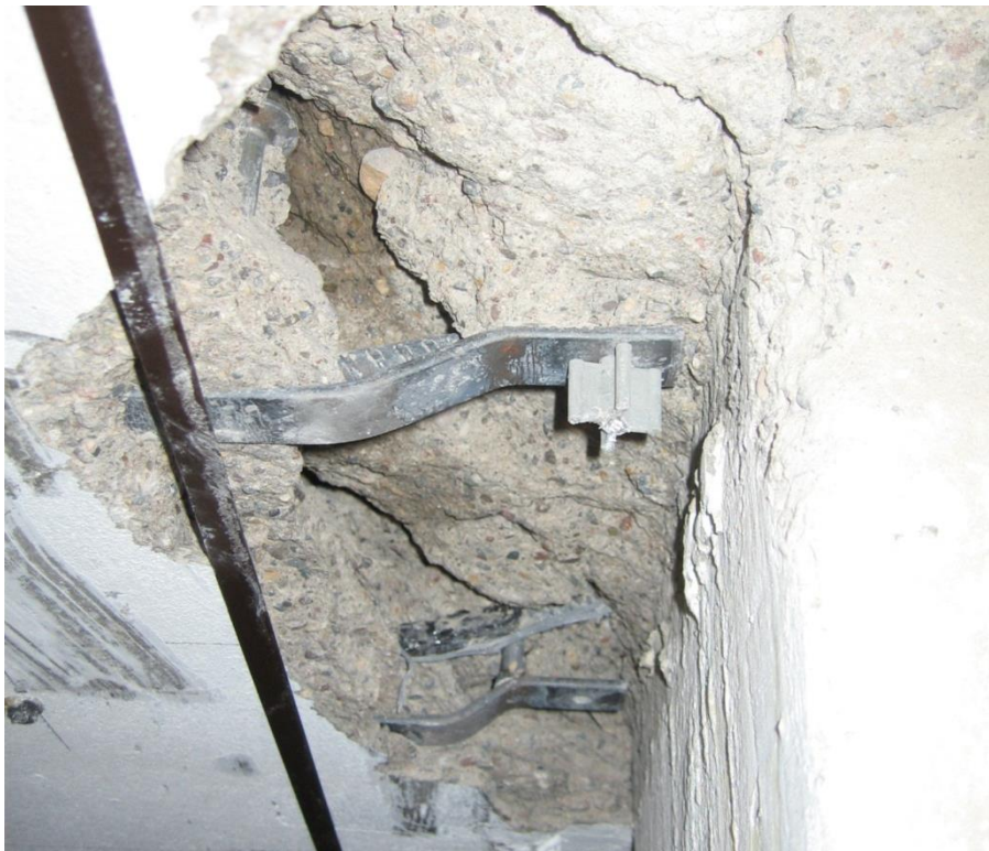
Figure 1-6: Punching Shear Crack between First and Second Row of Shear Stud from Specimen SB3 (Cheng et al. 2010)
