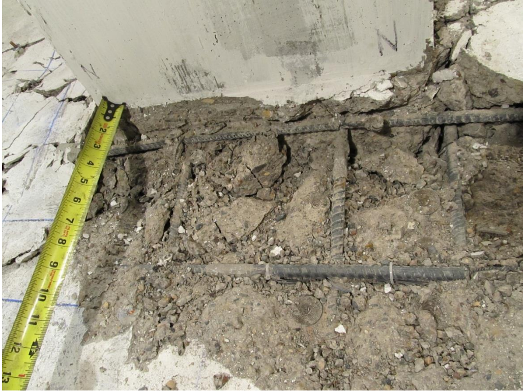
Figure 3-20: Specimen B4 – Gravel-Like Concrete within Connection Region
