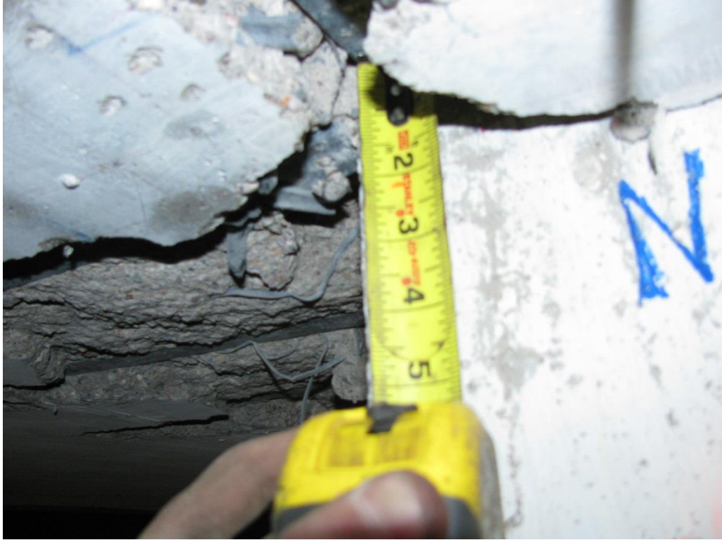
Figure 3-12: Specimen B1 – Bottom View of North-East Corner of Slab-Column Connection After Test
