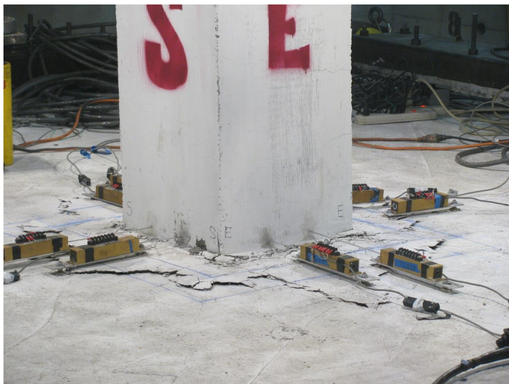
Figure 3-10: Specimen B4 – Connection Damage at 2.30% Drift, Point 8
