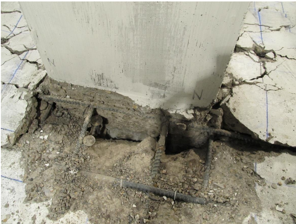
Figure 4-26: Specimen B4 – Void between Slab and Column after Loose Concrete Had Been Removed
