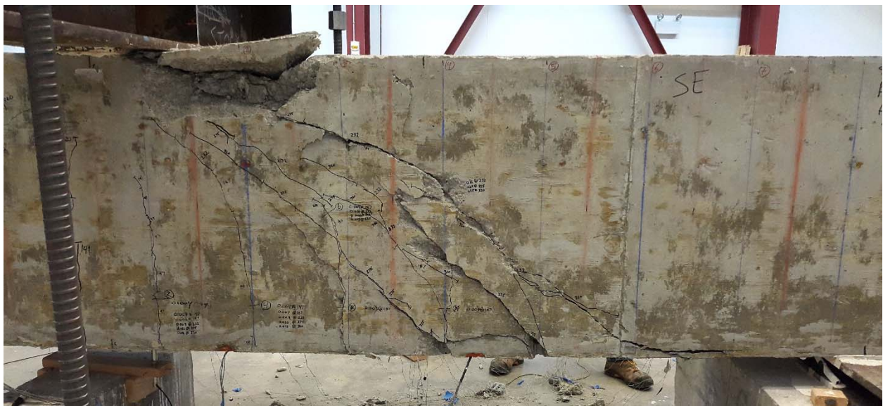
Figure 1.2: Inclined cracks in a reinforced concrete beam
