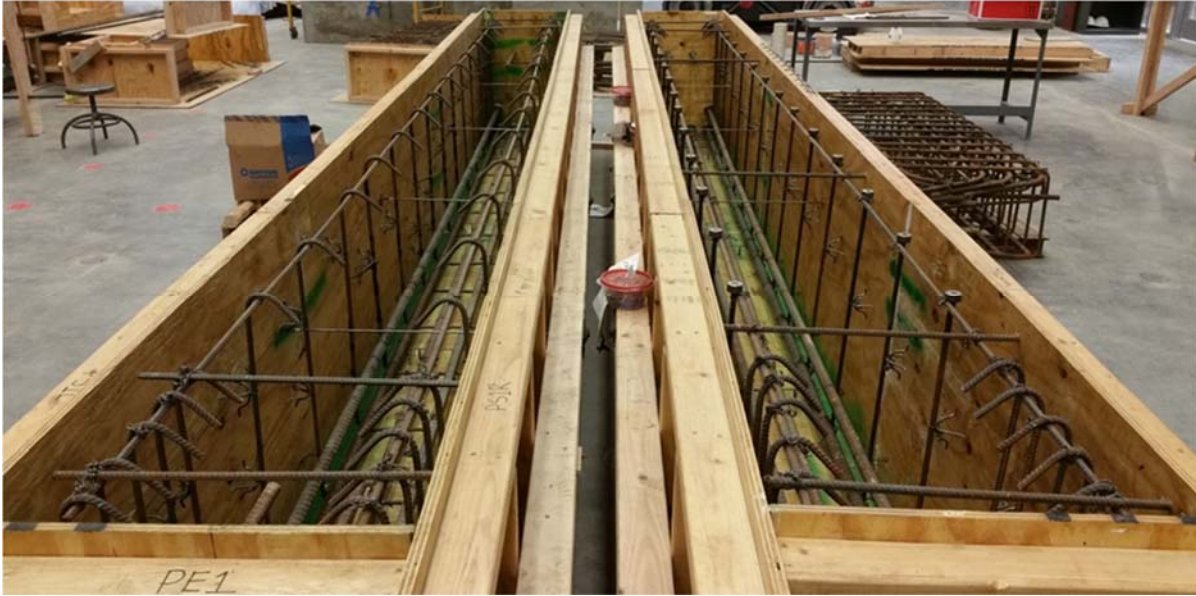
Figure 1.8: Reinforcement cages with conventional stirrups (left) and headed bars (right) as shear reinforcement
