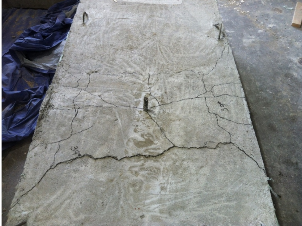
Figure 3.1b Breakout failure of slab specimen 8-5-F4.1-6#5-6 from test Series 5 with both supports outside the failure region (specimen contained a single bar anchored at the middle of the slab)
