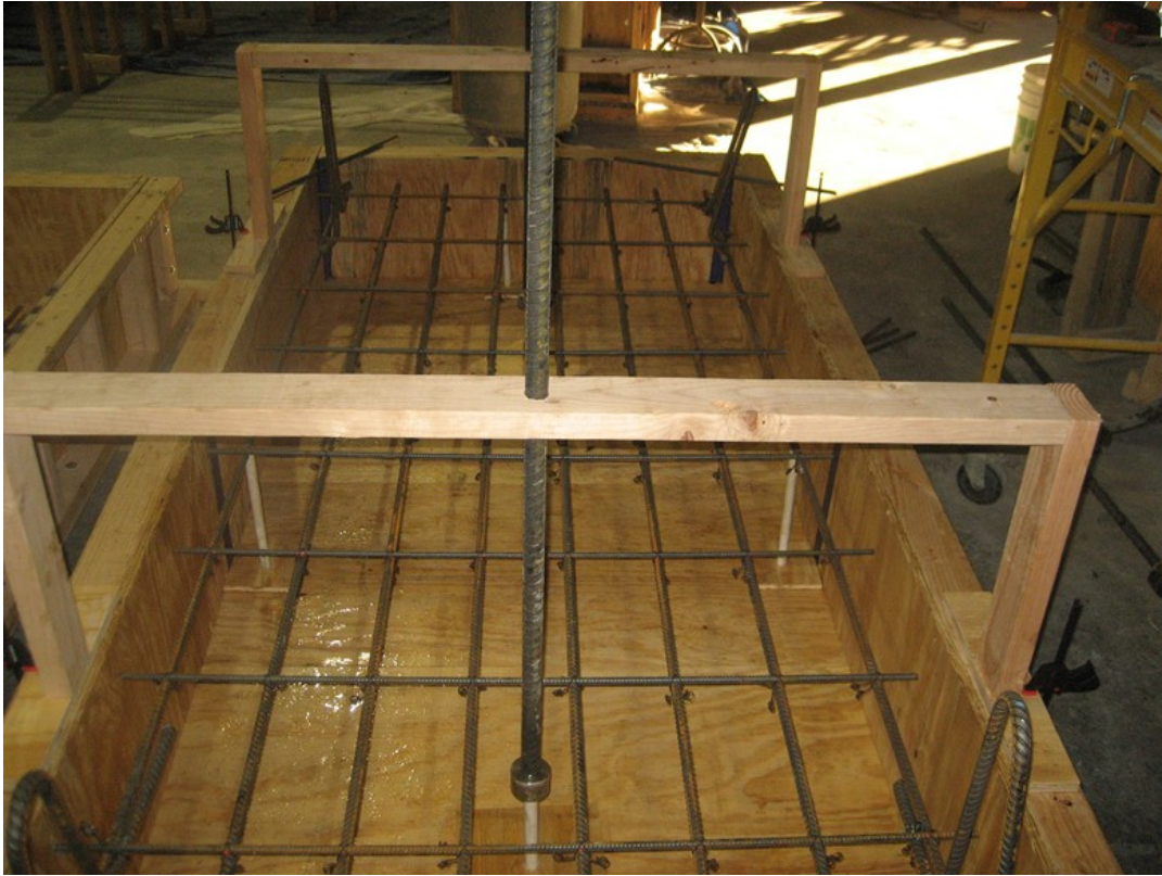
Figure 3.6 Slab specimens in Series 1 and 2 that contained No. 4 and No. 5 bars perpendicular to the headed bar distributed evenly along the long and short direction of the specimen
