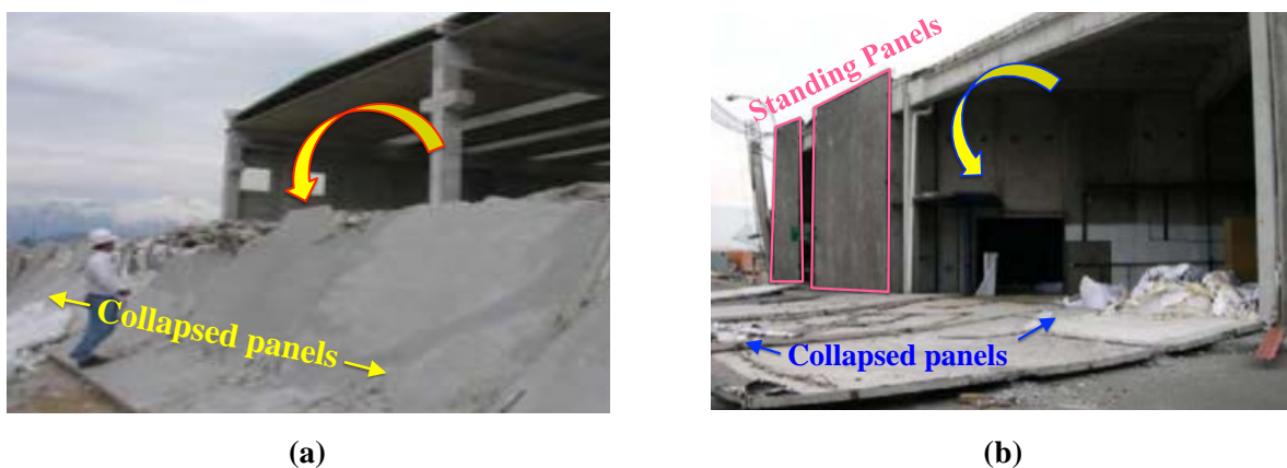
Figure 2.3. Photographs showing examples of collapsed panels after (a) the 2009 L'Aquila earthquake (Miyamoto International, 2009) and (b) the 2010 Chile earthquake (Gosh and Cleland, 2010)
