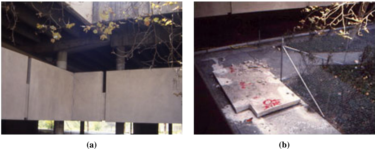
Figure 2.2. APC panel (a: as installed before) and (b: fallen from a parking garage) at CSULA during the 1987 Whittier Earthquake. One person was fatally wounding (Arnold, 2009 after Taly, 1988).
