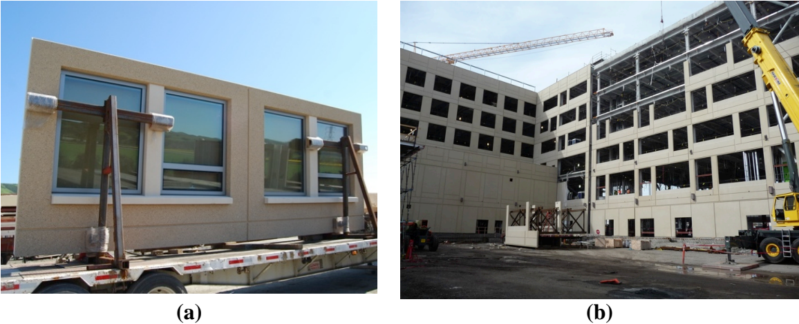
Figure 1.2. Examples of typical precast concrete cladding systems installed in the field: (a) punched panel system in transport and (b) u-shaped panels during installation.
