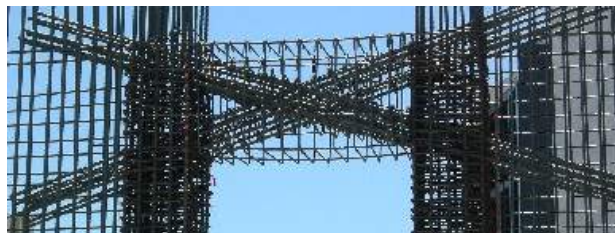
Figure 1.2: Diagonally-Reinforced Concrete Coupling Beam (photo courtesy of NEESR at the University of Michigan)
