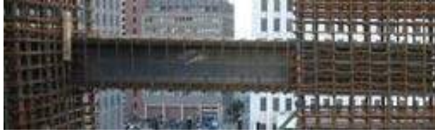
Figure 1.3: Steel Reinforced Concrete (SRC) Coupling Beam (photo courtesy of Magnusson Klemencic Associates)
