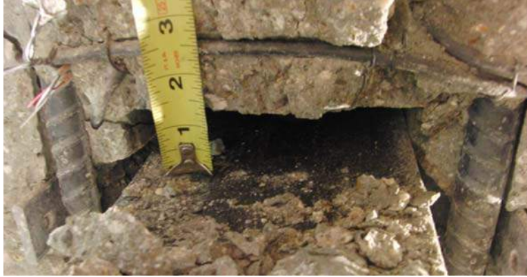
Figure 5.2: Photo Showing Gapping Between Steel Flange and Concrete (SRC2)
