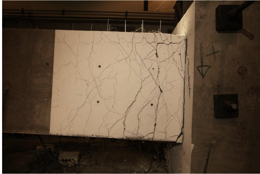
Figure 21 Beam 2: damage state during the second cycle with a peak drift ratio of 2.9% (instantaneous drift ratio = -2.0%).
