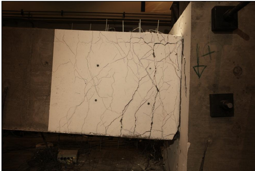
Figure 22 Beam 2: damage state during the second cycle with a peak drift ratio of 2.9% (instantaneous drift ratio = -2.9%).
