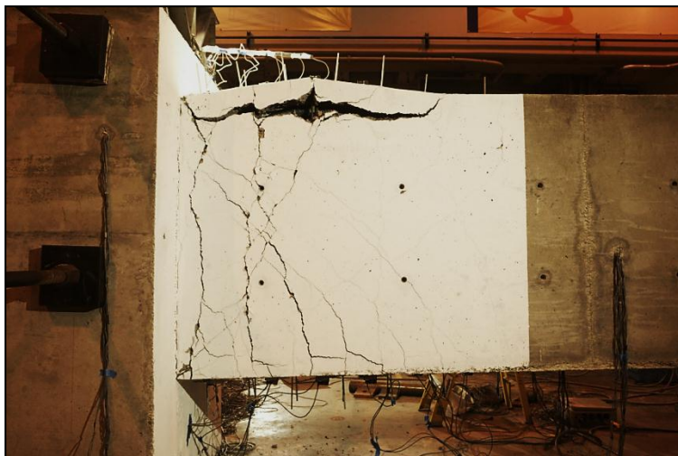
Figure 9 Beam 1: buckling of the top longitudinal bars (first cycle with peak drift ratio = 2.7%, instantaneous drift ratio = -2.7%).
