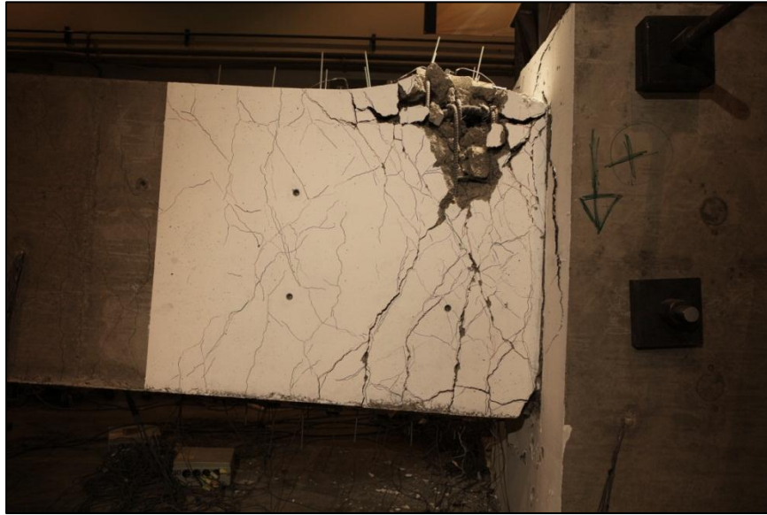
Figure 25 Beam 2: buckling of the top longitudinal reinforcement (first cycle with peak drift ratio = 3.9%, instantaneous drift ratio = -3.9%).
