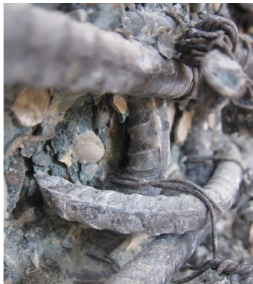
(e) west face ruptured CWT leg at the first bar north of the center bar
