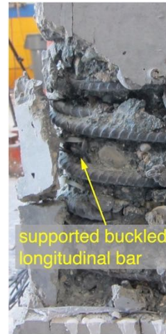
(f) south face damage
