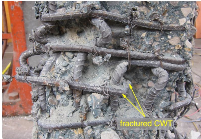
(e) damage and transverse reinforcement fracture on north face
